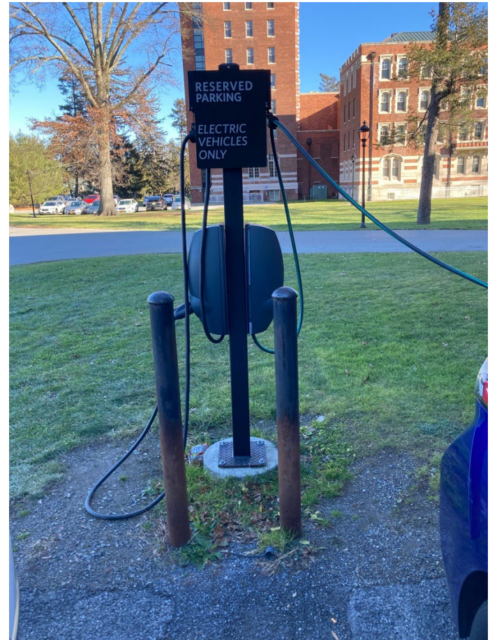
Pair of chargers at Vassar College (Note that the post is taller and painted brown, bollards have their own foundation, and sign is similar our signage)
