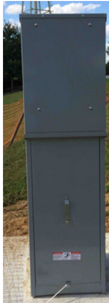
Peppo meter cabinet (Should be screened)
